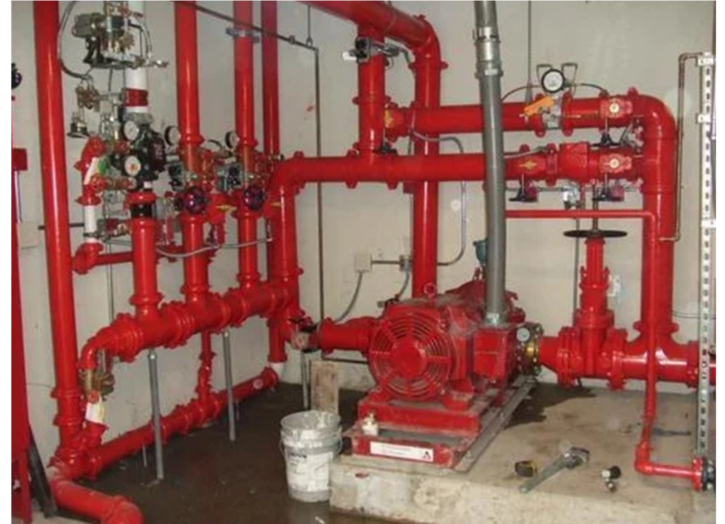
Electric Motor Driven Fire Pump
