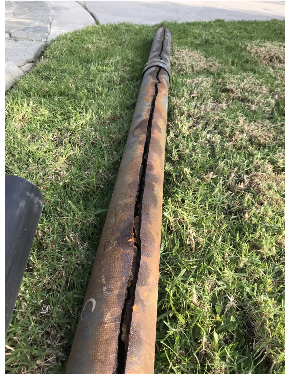
Typical Tru Spun Pipe Failure
